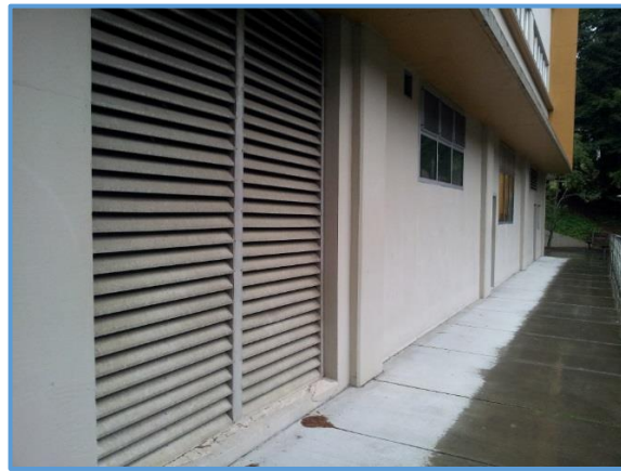
Figure: 17 Air vents on the south side of Science A
